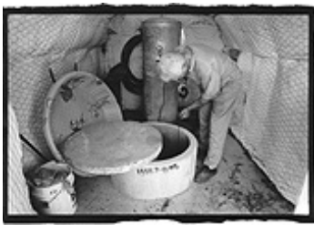
Figure 10. Harold Fain checks his 37-foot well near the Ozarka tract. Biggest Pump Wins (photograph by Mark Graham).
